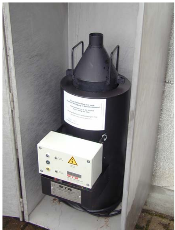
Wechselfilter in Regenerationsanlage
